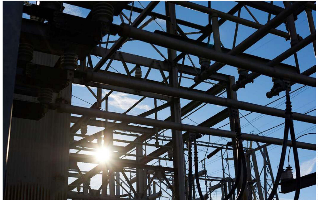
Generic Substation Photo
