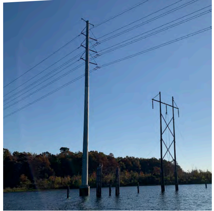
Williams – Goose Creek 230KV/115KV, Williams – Faber Place 230KV Transmission Lines
