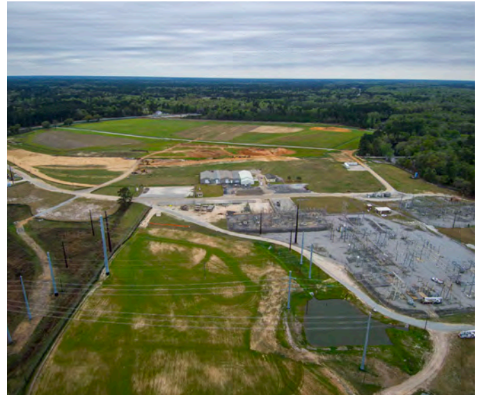
Existing Canadys 230KV/115KV Substation located on the Canadys brownfield site
