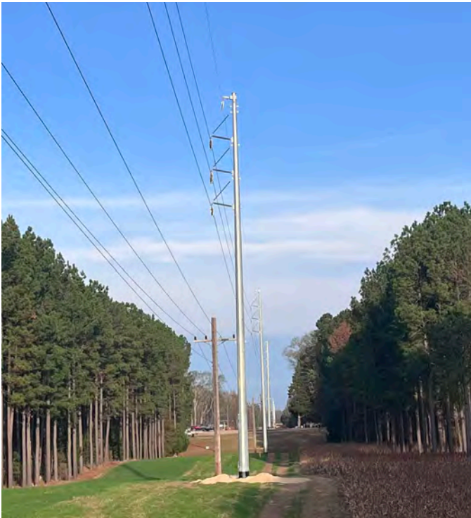
Batesburg – Saluda County 115KV Transmission Line
