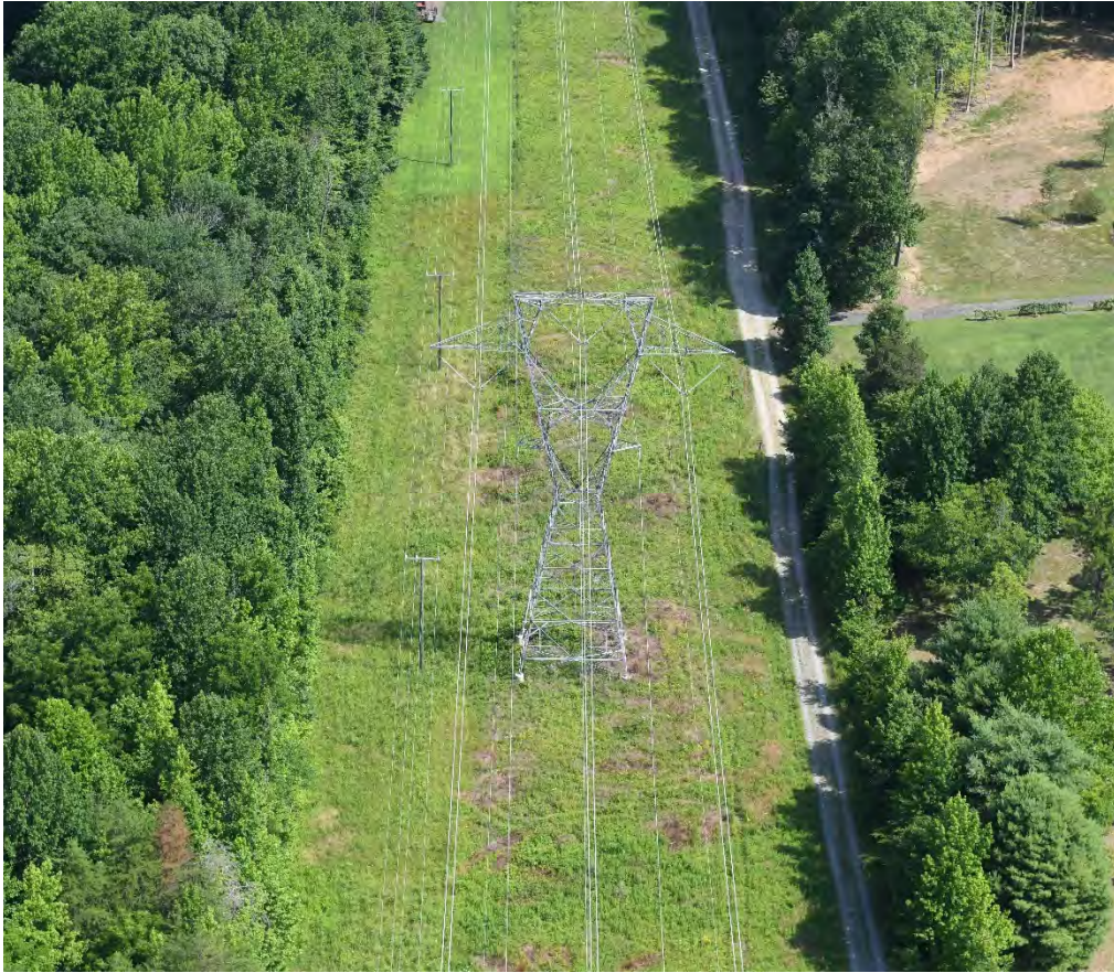
5-2T Double Circuit Suspension Tower
