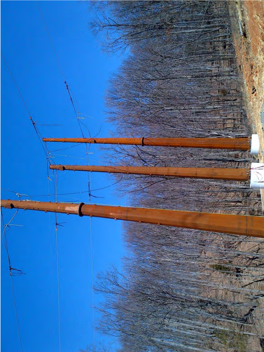
Typical 3-Pole Structures
