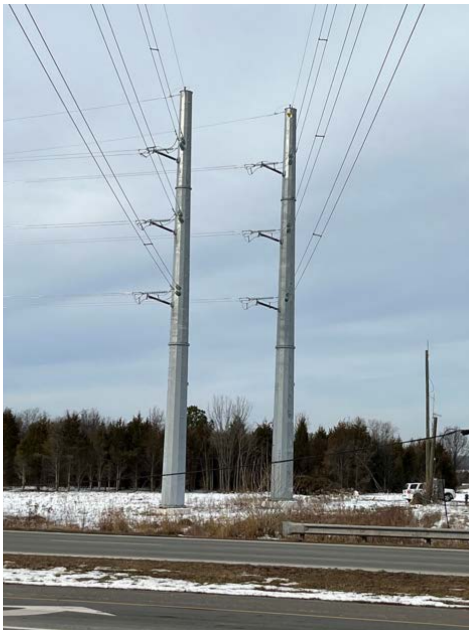
Double Circuit Engineered 2-Pole Double Deadend Structure
