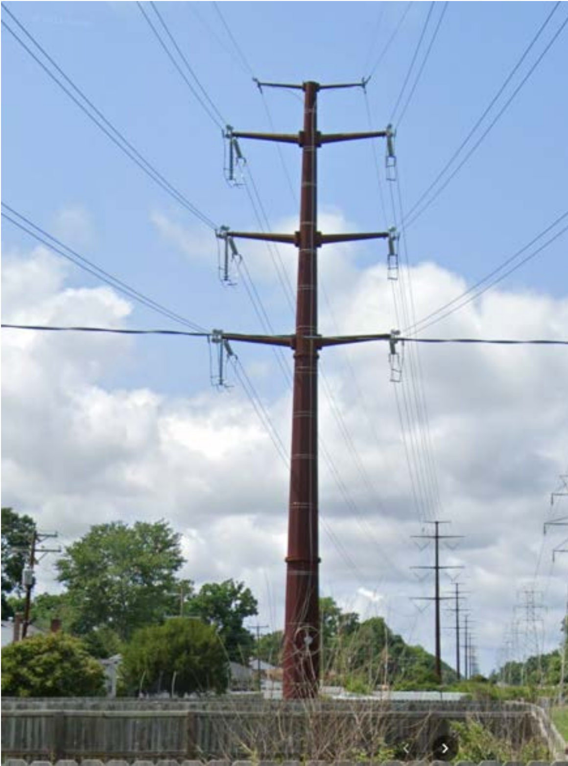
Double Circuit Engineered Monopole Double Deadend Structure
