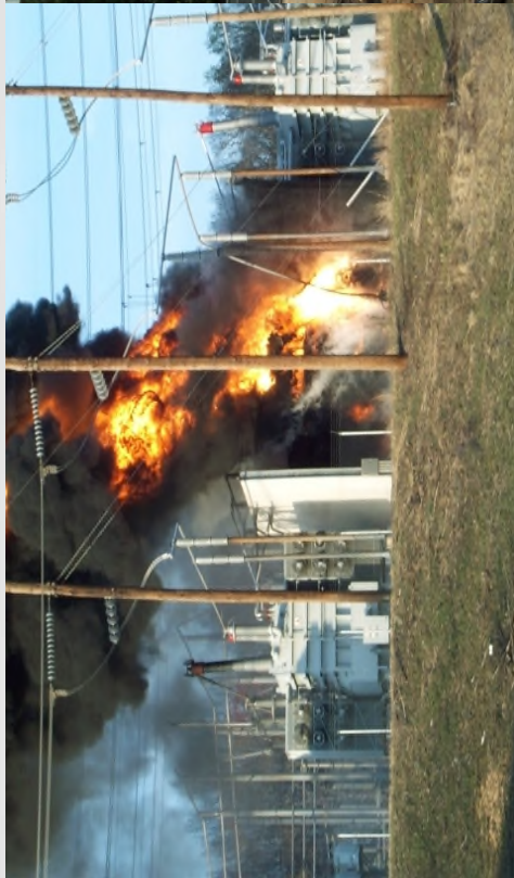
500 kV Transformer Failure in 2000
