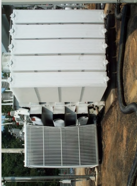
230 kV Transformer Failure in 2001
