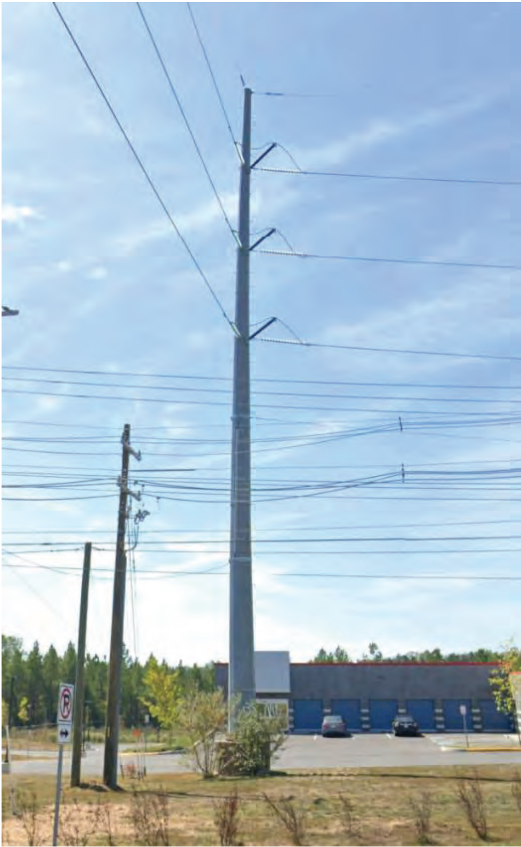
Proposed Structure Type: 230 kV Single Circuit Steel Monopole (DDE - No Conductor Arms)
