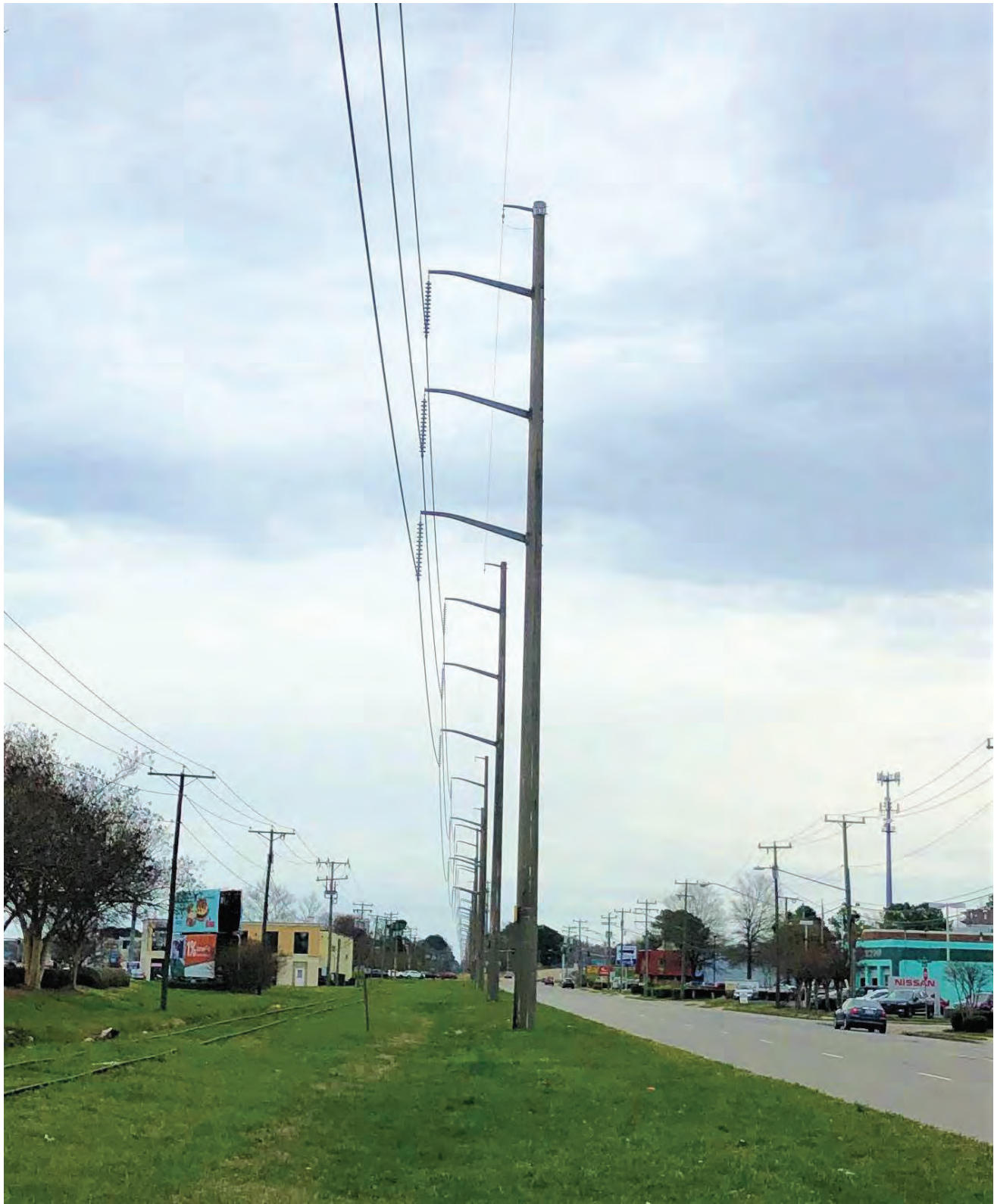
Existing Structure Type: 230 kV Single Circuit Concrete Monopole (I-String Suspension)
