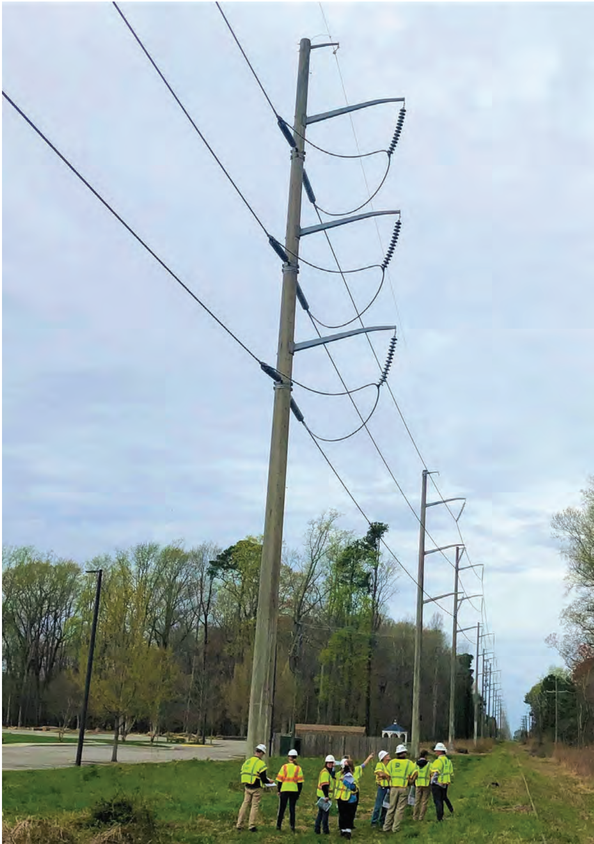
Existing Structure Type: 230 kV Single Circuit Concrete Monopole (DDE - With Conductor Arms)
