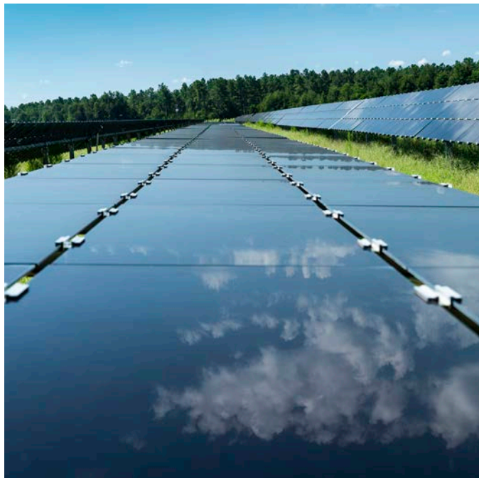
Springfield Solar Farm; Springfield, VA.
