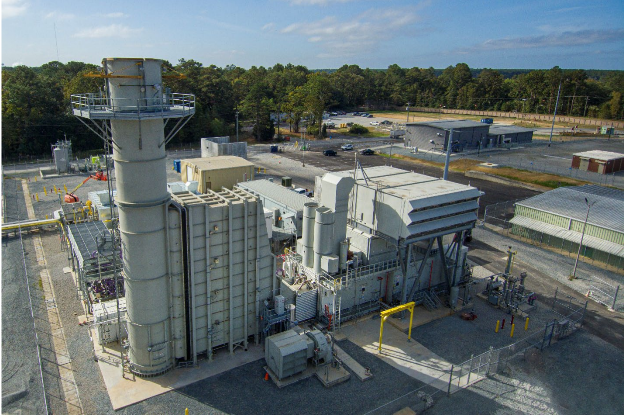
Figure 3: Bushy Park CT #1 Unit (In Commercial Operation)
