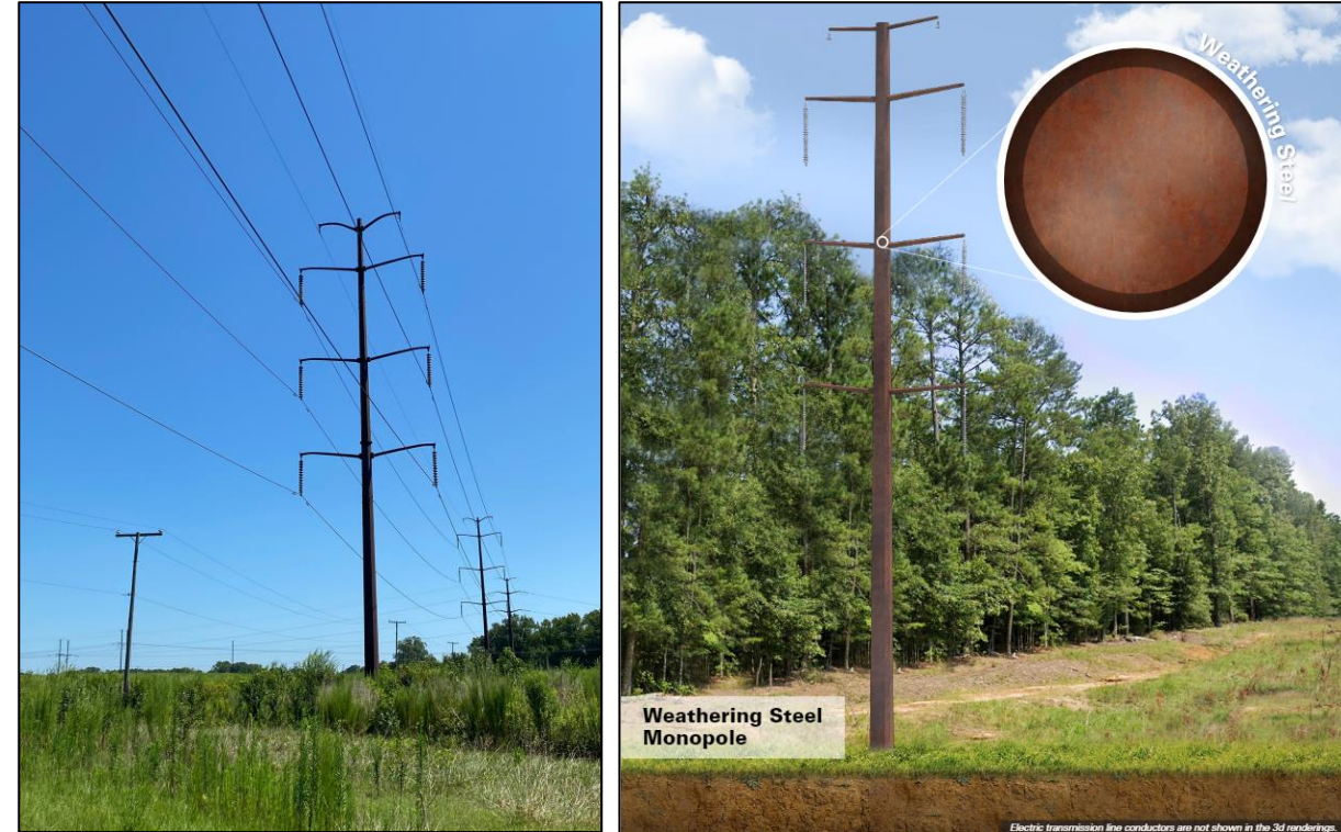
Examples of electric transmission double-circuit monopole structures. Not project specific.
