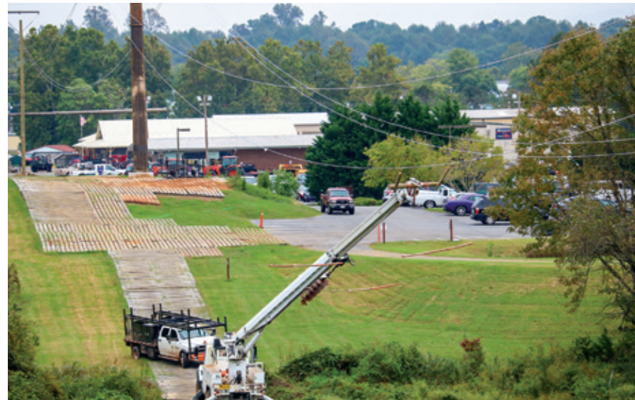
Wooden matting is placed to protect the right of way corridor during construction. After construction is completed, crews remove the matting and begin restoration of the right of way.
