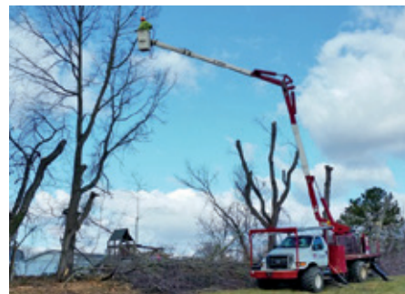
Right of way clearing involves removing trees to maintain minimum clearances between vegetation and transmission lines.
