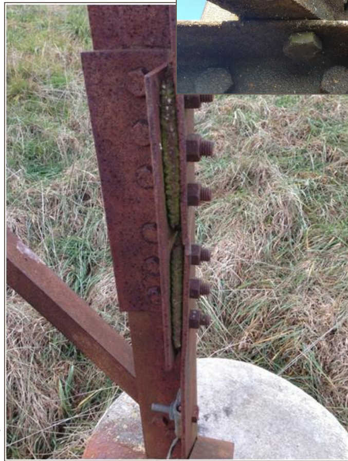
Representative pictures of aging structures.
