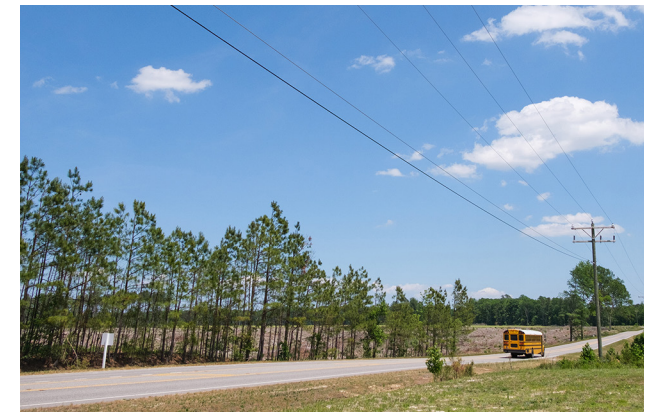
The fiber optic cable is the lowest line on this span.
