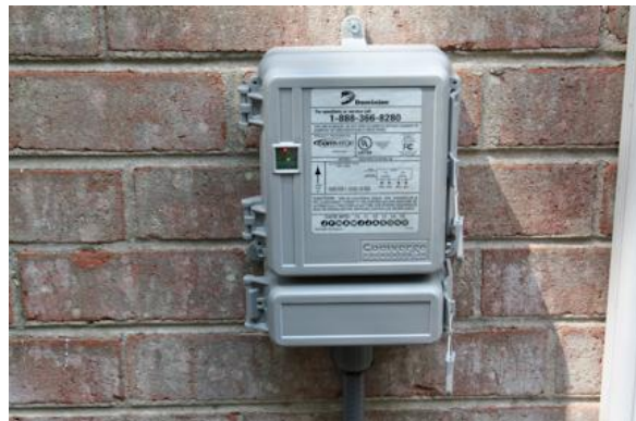
AC Cycling Switch Installed
